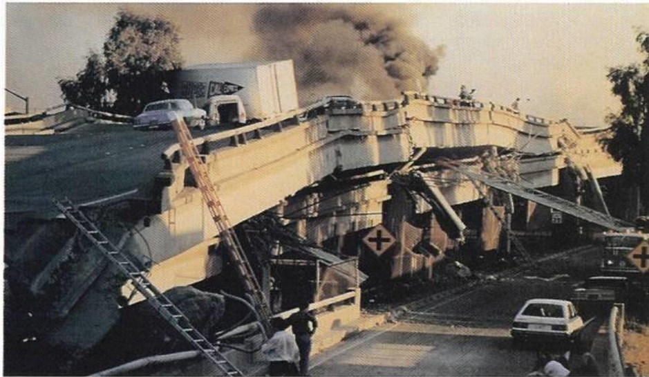
Figure 3-22 This collapsed California highway is evidence of the tremendous energy unleashed during an earthquake.
