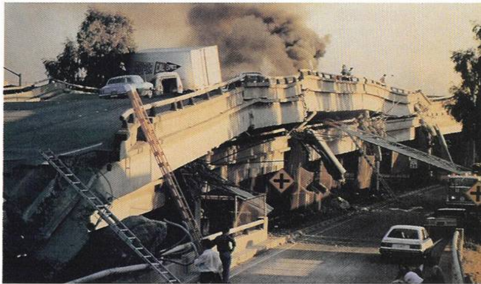
Figure 3-2: California highway collapsed during an earthquake.
